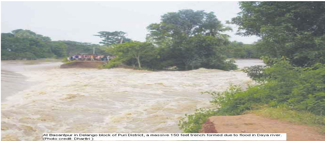
At Basantpur in Delango block of Puri District, a massive 150 feet trench formed due to flood in Daya river. (Photo credit: Dharitri )
